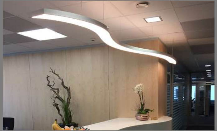
Backlit aluminum structures - Light Fixture - Switzerland Application : Linsi-tech
